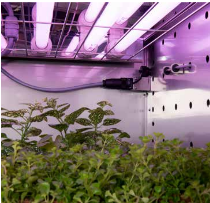
Interior of Forma Vertical Light Chamber with plant growth light modules installed.
